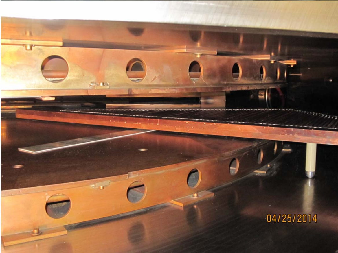
FIG. 2. Top – Cryopanel for the K150 cyclotron. Bottom – Installed cryopanel in the K150 cyclotron. The cryopanel is stood off from the trim coil cover with three feet, one is very short near the center of the cyclotron, and two others are at outer radii.
